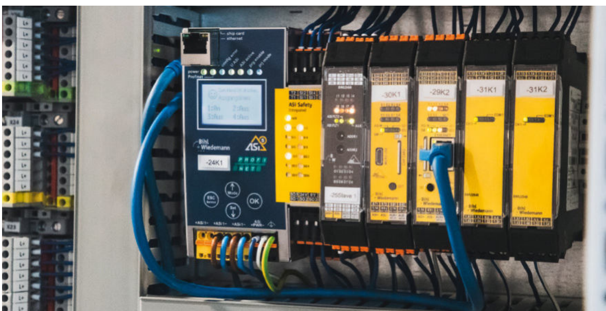
Safety technology in the control cabinet: ASi Safety Gateway (left) and Safety Basic Monitors (center) from Bihl+Wiedemann.
