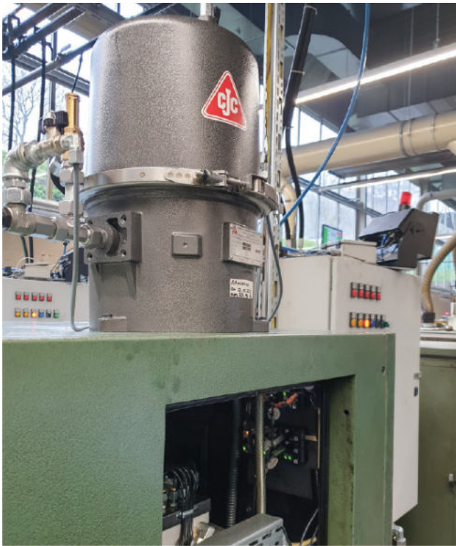
Process and diagnostic data from IO-Link sensors for pressure, temperature and flow can now be used in ASi-5 for predictive maintenance.
