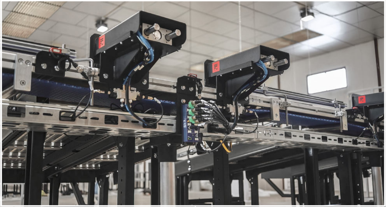
Using the ASI-5 self-configuring I/O modules BWU4231 from Bihl+Wiedemann, optical sensors and pneumatic actuators are integrated for the ejection of packages.
