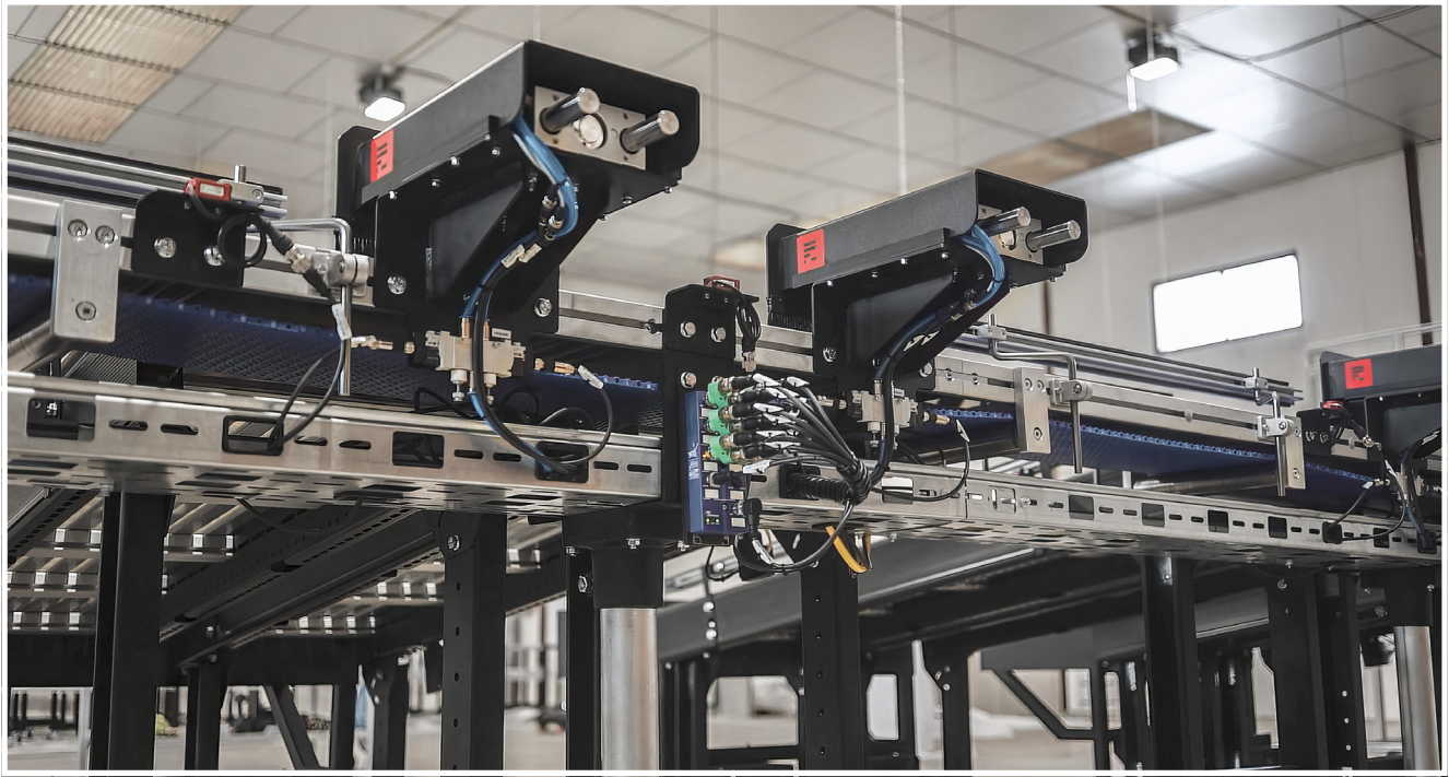
Using the ASI-5 self-configuring I/O modules BWU4231 from Bihl+Wiedemann, optical sensors and pneumatic actuators are integrated for the ejection of packages.
